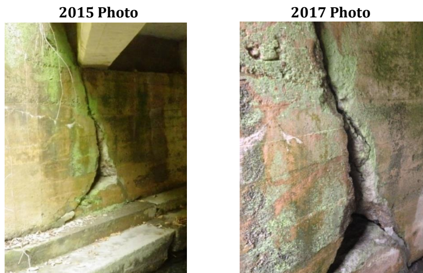
Figure 8: Crack in Randolph Bridge #36 Abutment
