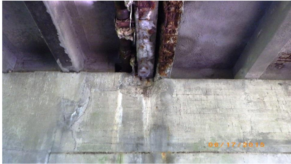
Figure 5: Example of Concrete Deterioration on a Municipal-Owned Bridge
